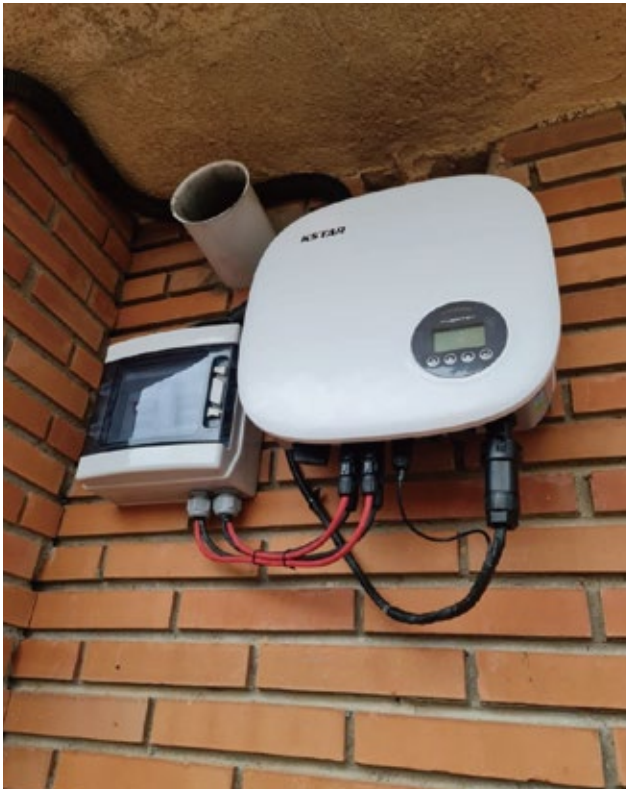
06 Residential Solar Project in Brazil
