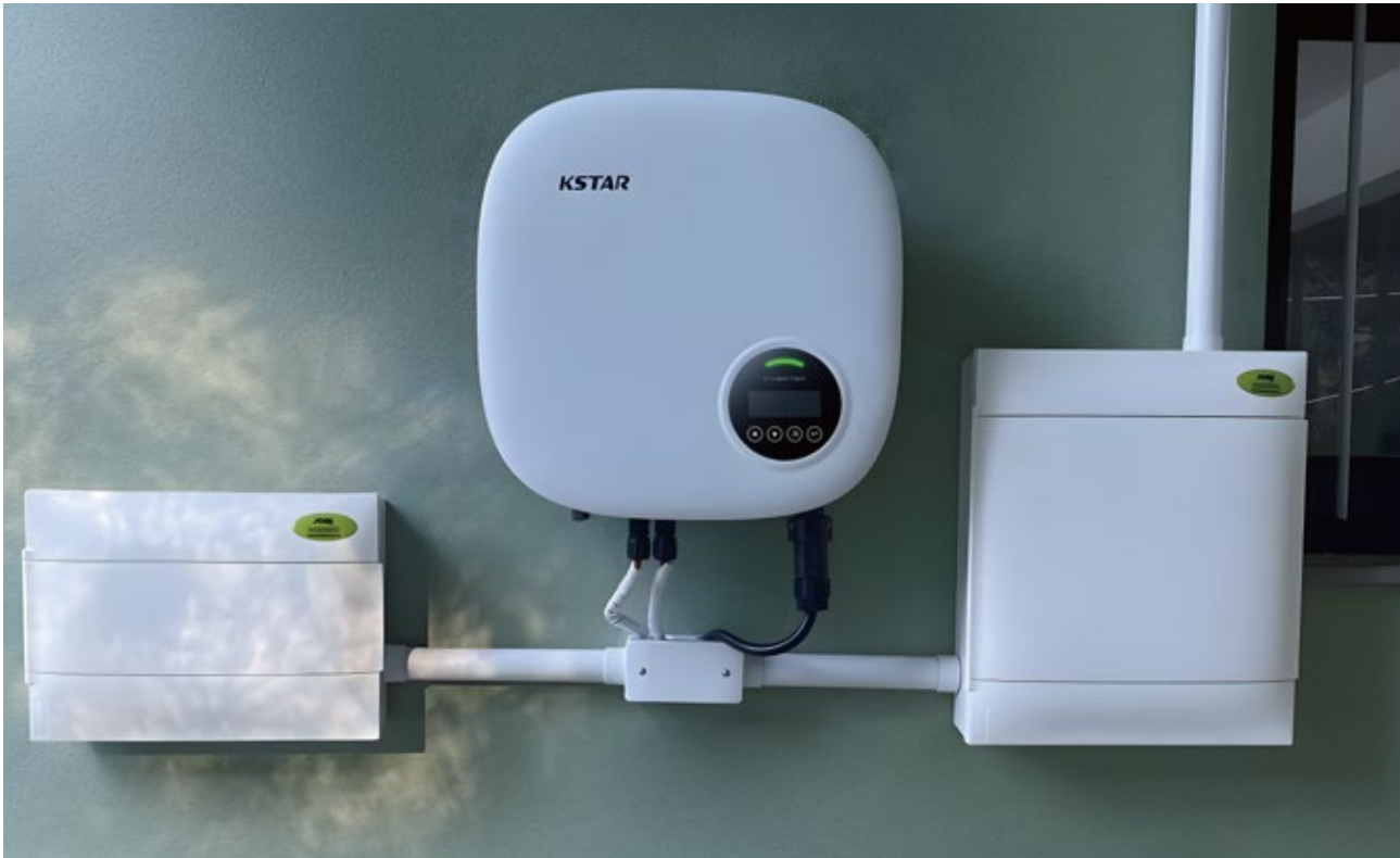
09 Residential Solar Project in Brazil
