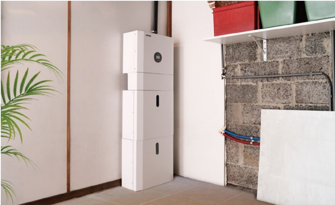
08 Residential ESS Project in the Netherlands
