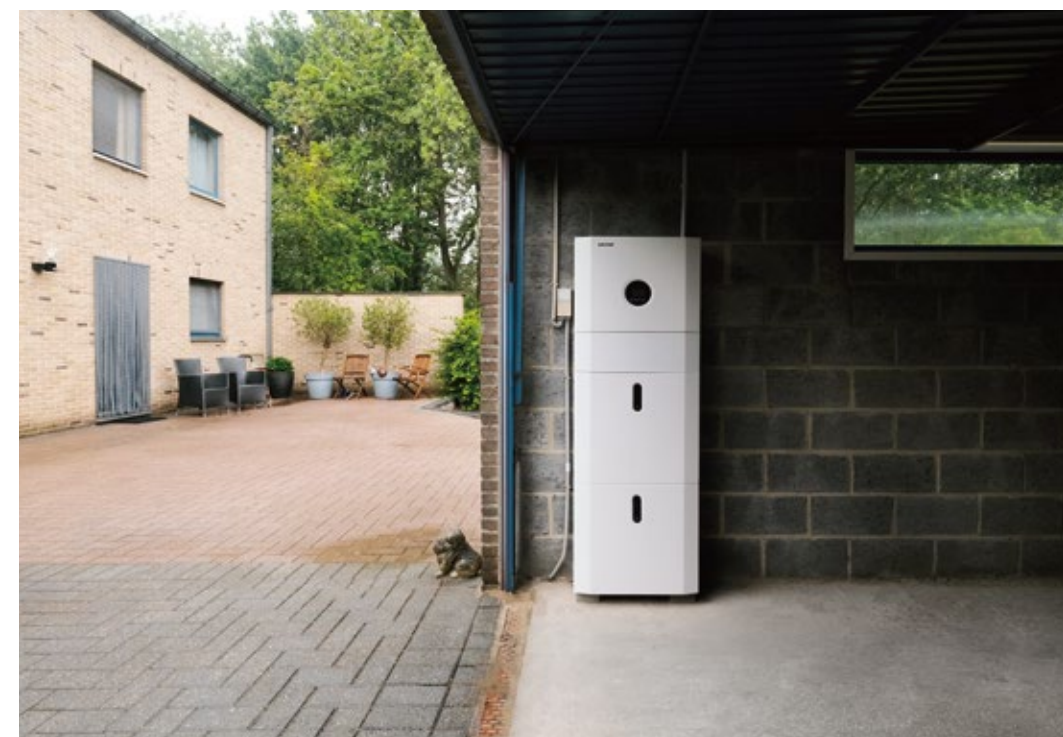
04 Residential ESS Project in Belgium
