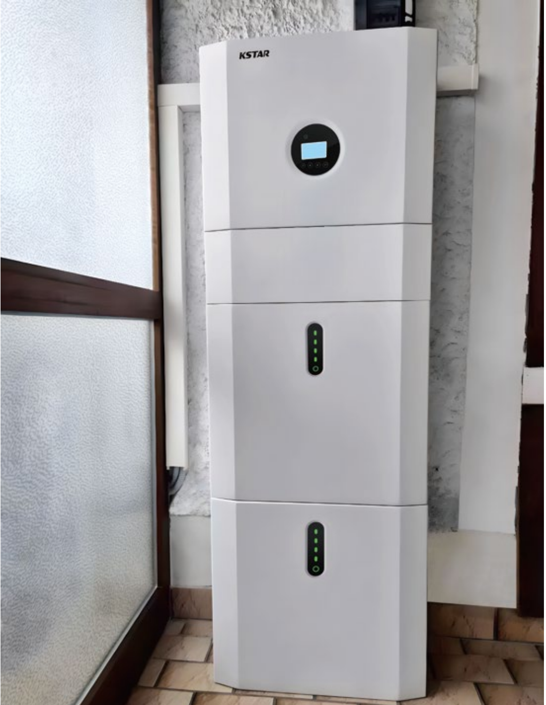
11 Residential ESS Project in Italy
