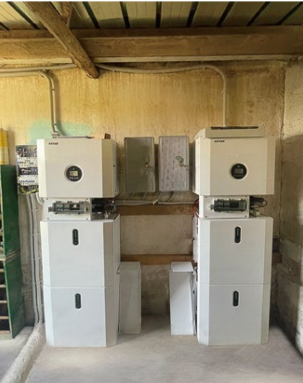
07 Residential ESS Project in Italy
