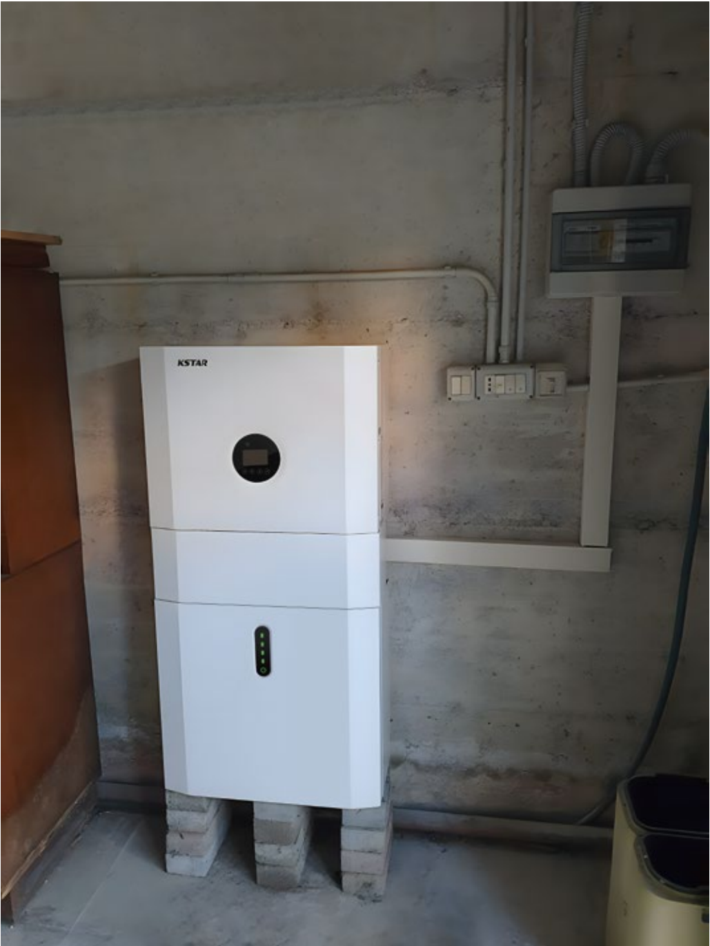
10 Residential ESS Project in Italy
