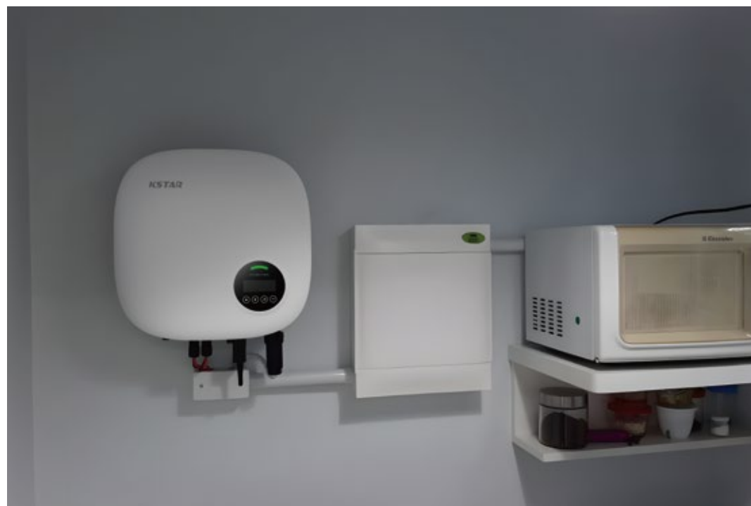
03 Residential Solar Project in Brazil
